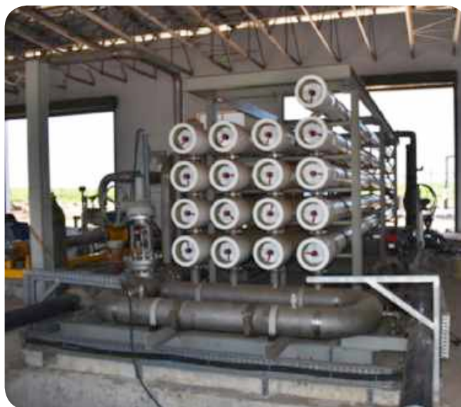
Vipingo Development Limited desalination plant
