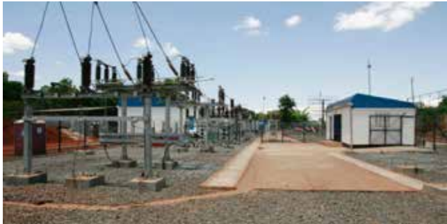
Two Rivers substation
