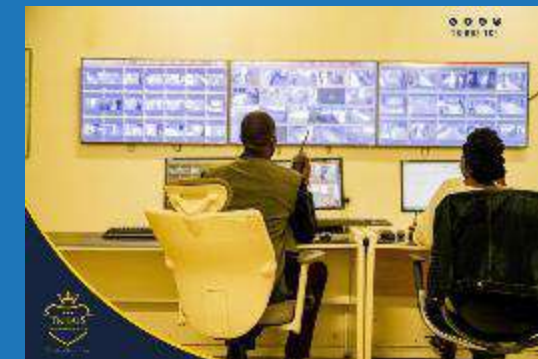
Security Operations Center
