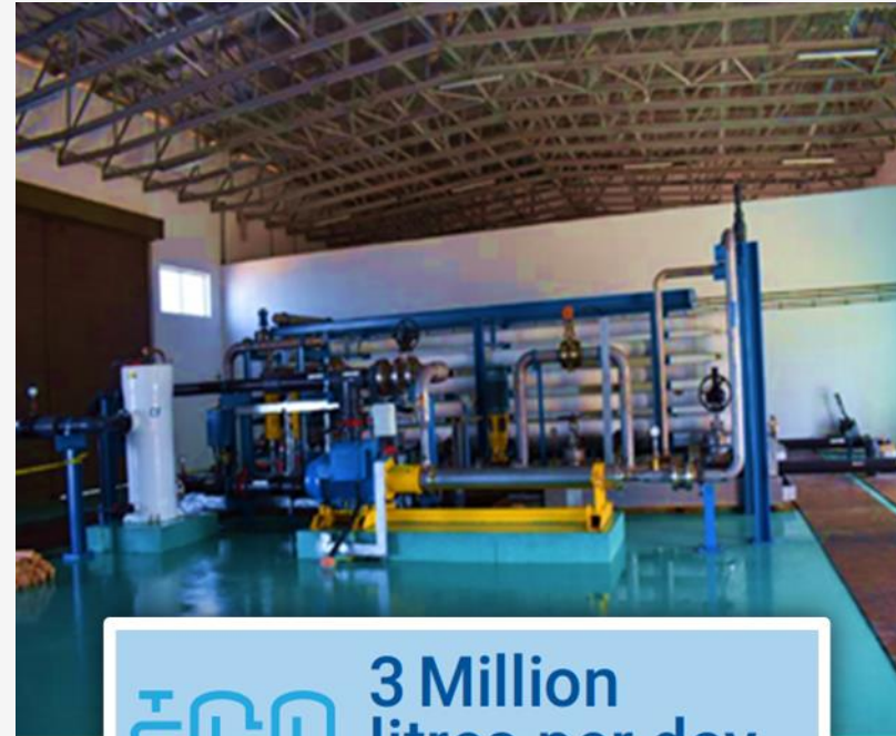
Newly installed reverse osmosis desalination plant
